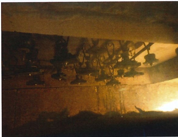
Figure A4.2 View of the clamps in the 10th minute of test.
