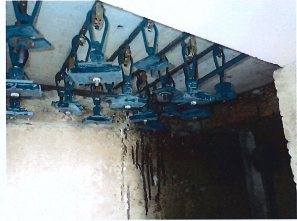
Figure A4.7 View of the clamps after the fire test.
